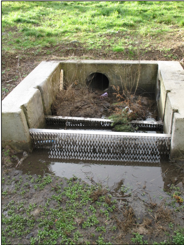
Sediment Trap with Accumulated Sediment
