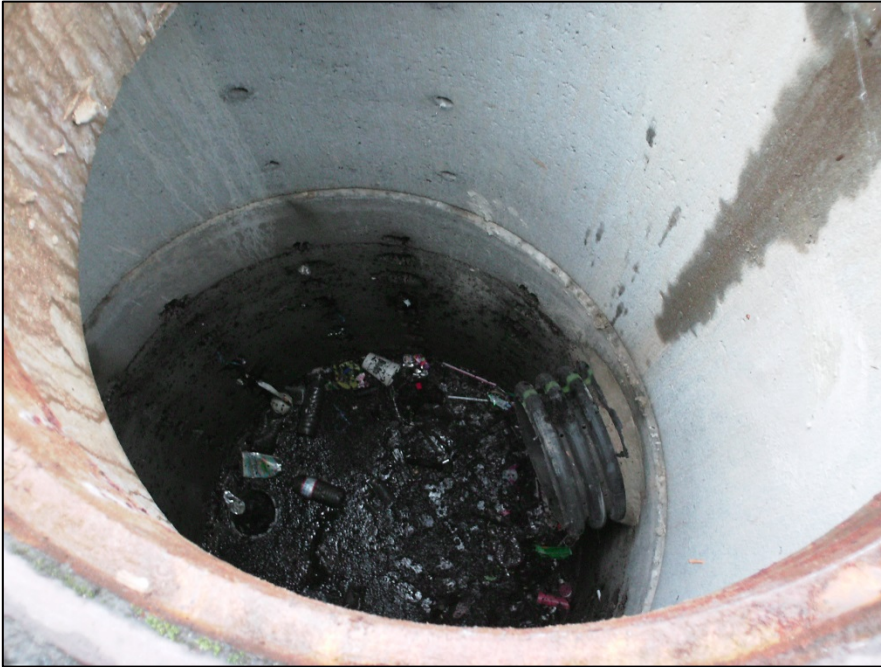
Drywell with Accumulated Trash
